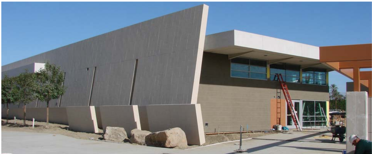
Public Safety Academy: Workmen put finishing touches on the Public Safety Academy at Palm Desert, located in the northeast corner of the COD campus. The two buildings shown here will anchor a facility that includes classrooms as well as outdoor exercise and training facilities. The PSA facility will be the training center for all future police officers and firefighters in the eastern portion of Riverside County, which includes all of the Coachella Valley.
