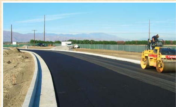
Site Prep for East Valley Modular Village: Work will be completed in time for a Spring 2009 semester opening of the interim East Valley Campus of COD, located at Avenue 62 and Buchanan Street in Mecca/Thermal.
